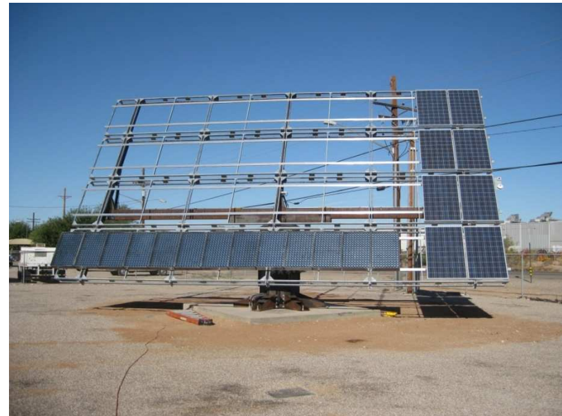
≈1.5kWp Rondine system, Tucson (US)
