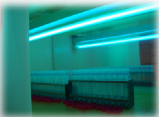
UV-irradiation of all disposables and working area
